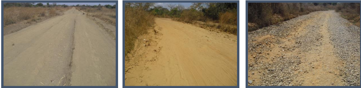
Picture: 3, 4 & 5. Some bad areas of the road and the stones put on parts of the road to alleviate the situation
