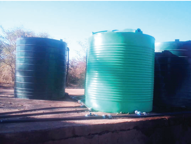
Figure 2: Installed water tanks
