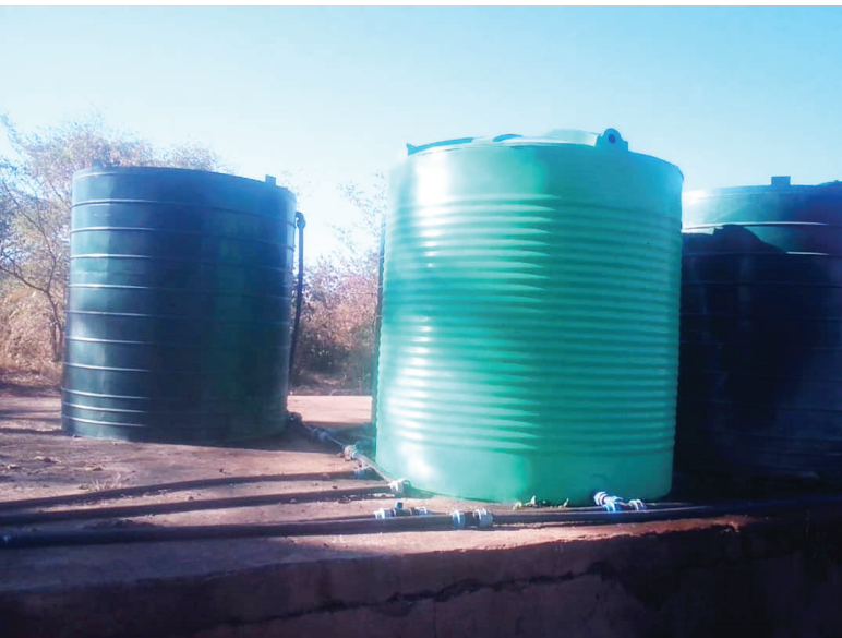
Figure 2: Installed water tanks
