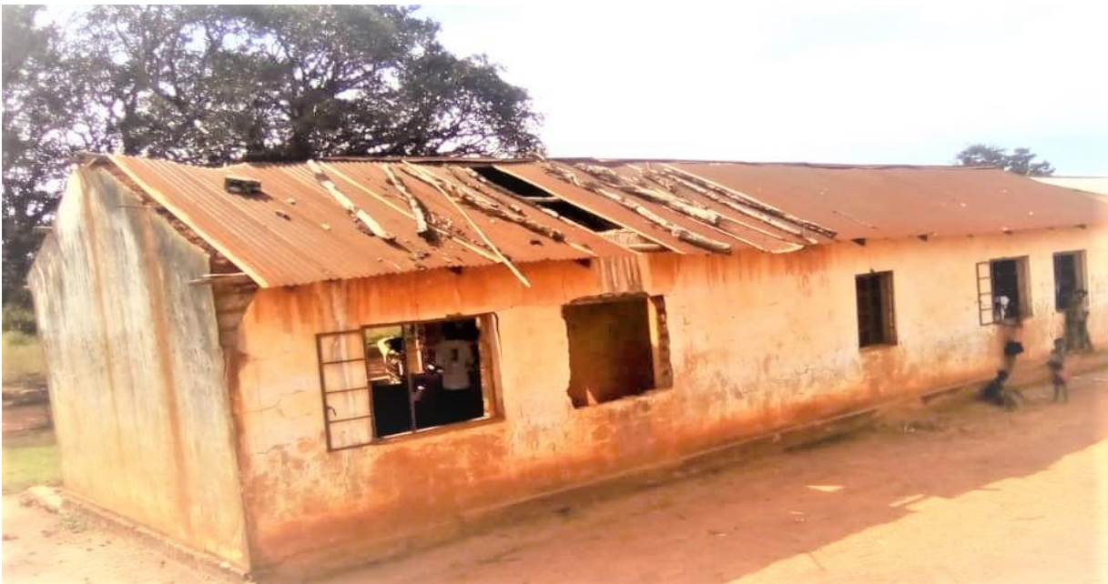
Image 4: Dilapidated classroom block at Chinemu primary school in Lufwanyama; JCTR 2021
