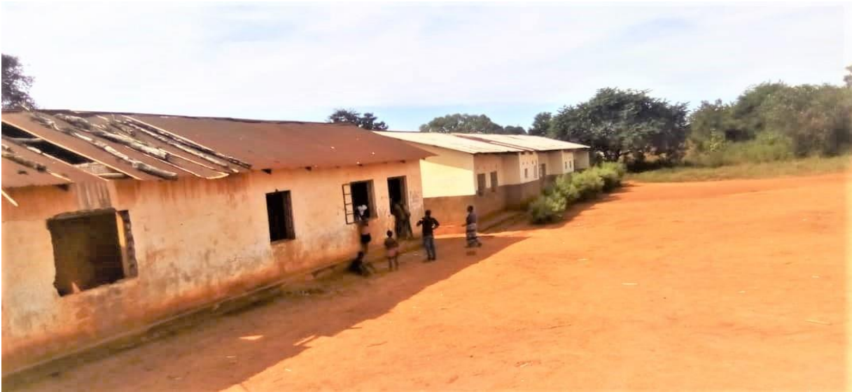
Image 3: Dilapidated classroom block at Chinemu primary school in Lufwanyama; JCTR 2021
