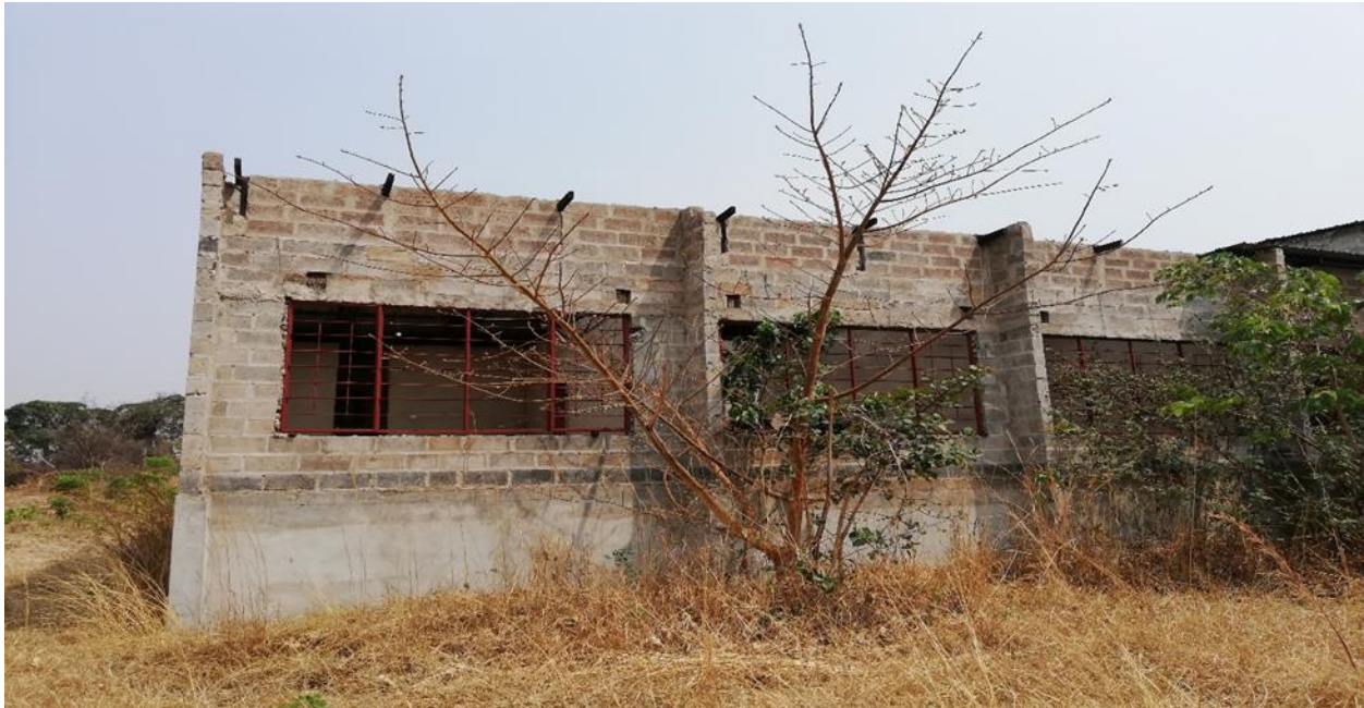
View of the blown roof
